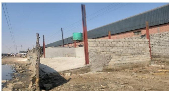
Incomplete Garbage Bay
