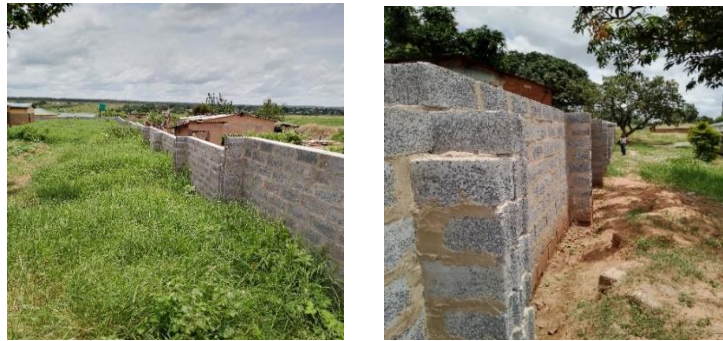
Incomplete wall fence
