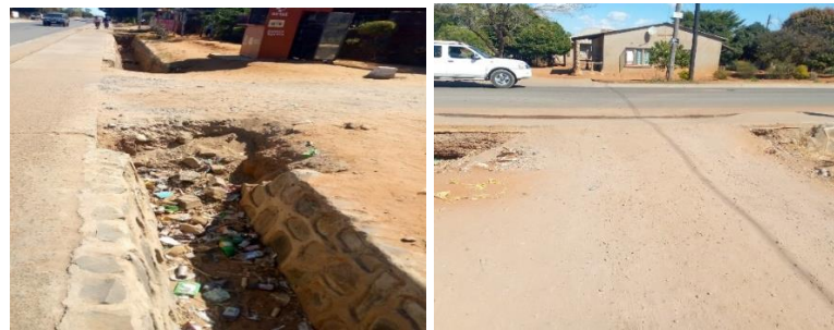
Crossing Points into Streets not done
