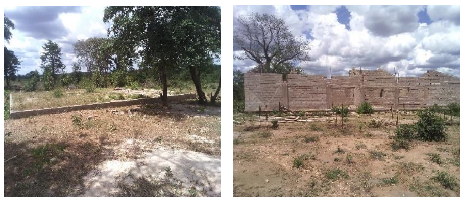
Incomplete works at Mtsanya Health post
