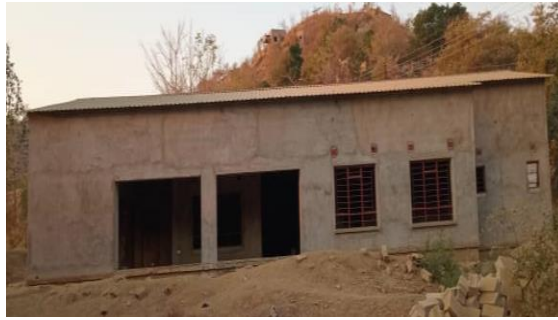
Incomplete Kaleya Clinic
