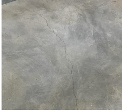
Cracks on the Floor
