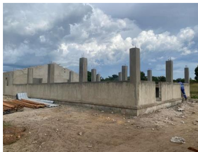
Uncompleted Market Shelter at Kalamba
