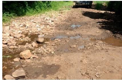
Water ponding at 1.6Km
