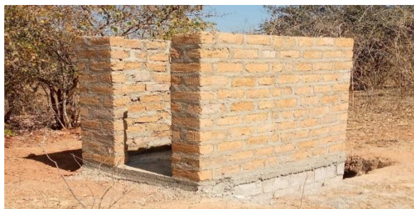
Incomplete VIP Toilet
