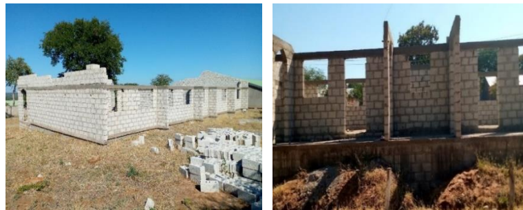
Stalled 1 x 3 Laboratory at Kazungula Secondary School Warped Pillars
