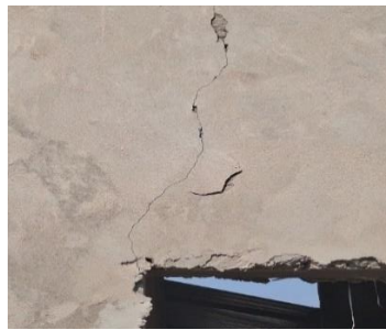
Cracked Plastered Wall
