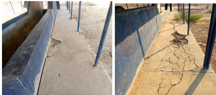
Poor workmanship – Construction of dip tank.
