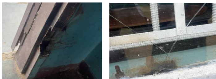
Door frame without a door Cracked window
