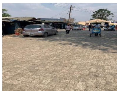
worn out pavers
