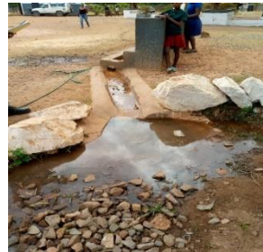
Soak Pit Overflowing at Mutamba Primary School
