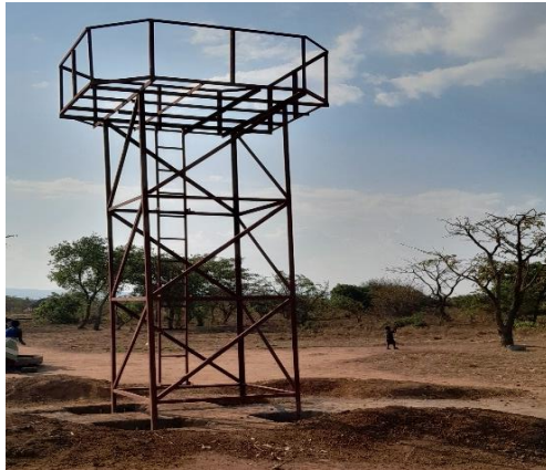
Incomplete water reticulation
