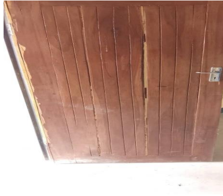
Cracked Soft Wood Door
