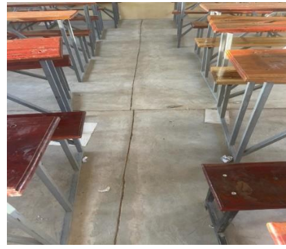
Expansion Gap not properly made
