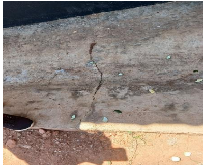
Cracks on the Spoon drainage
