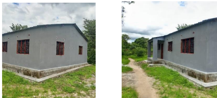
Incomplete Teachers House at Eden community house
