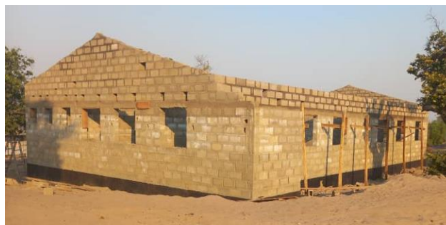
Incomplete Maternity Wing
