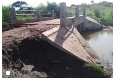
Eroded part of the bridge
