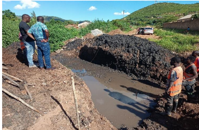
Delayed Completion of the Chizongwe Foot Bridge
