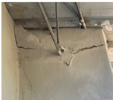
Cracked Concrete Padstone
