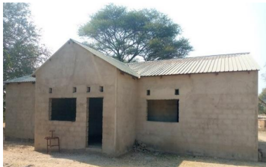
Stalled Project – Maamba Police Cells
