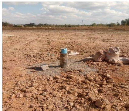
Uncomplete water reticulation system
