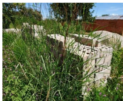
Unused Material on Site
