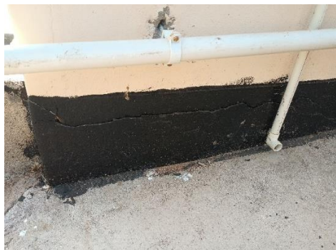
Cracks in the foundation box
