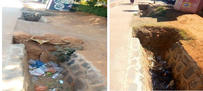
Crossing Points into Residents not done
