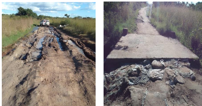
Uncompleted Rehabilitation of 14Km Road in Luchinde Ward
