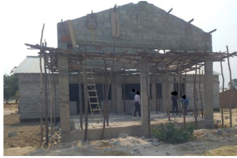
Incomplete Maternity Wing at Musele Health Post
