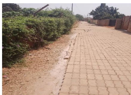
Incomplete Christon Tembo Road
