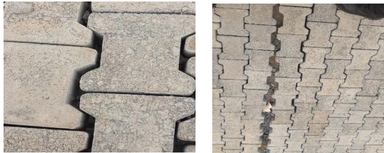
Failure to Lock Pavers
