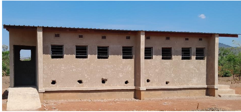
Incomplete ablution block
