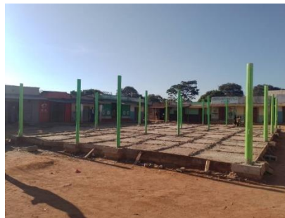
Incomplete market shelter
