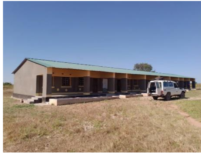
Incomplete Classroom block
