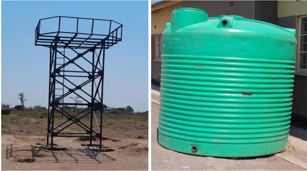
Tank Stand and tank marooned due to Incomplete works
