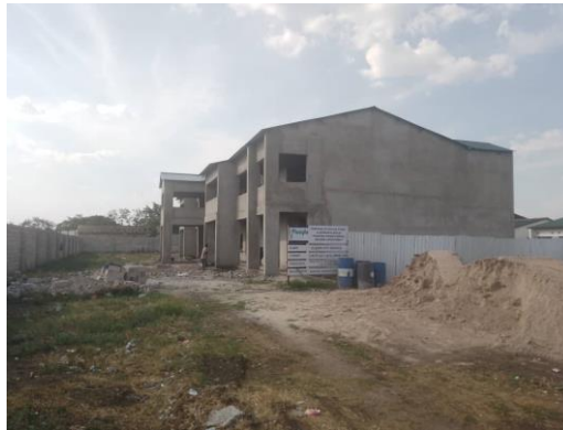
Twashuka Combined School Incomplete Structure
