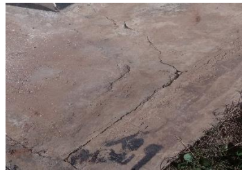
Cracked Spoon Drain
