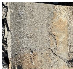
Crack on Spoon Drain
