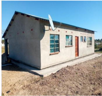
Air vents and glass Panes not fitted
