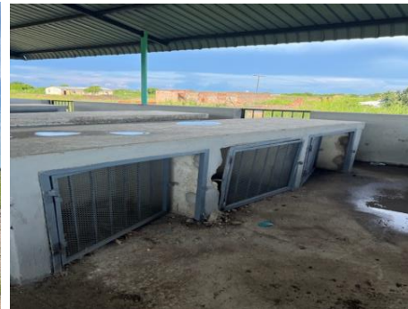
Vandalised Grill gates
