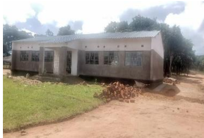
Incomplete classroom block
