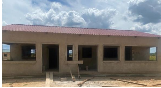
Uncompleted Kaoma-Ndonga Health Post
