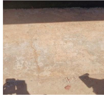
Cracks on Veranda
