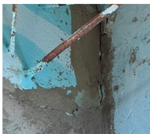
Crack on Concrete Pad
