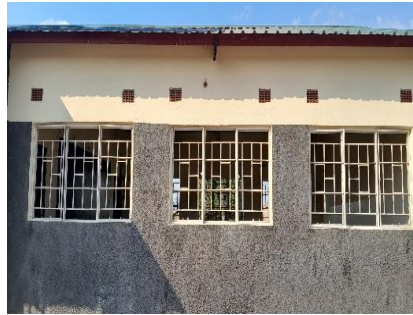
Windowpanes not fitted
