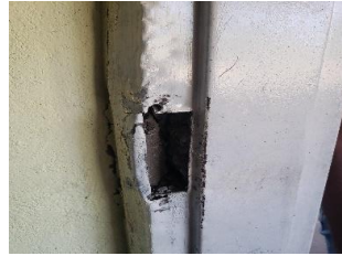
Poorly fabricated door frame
