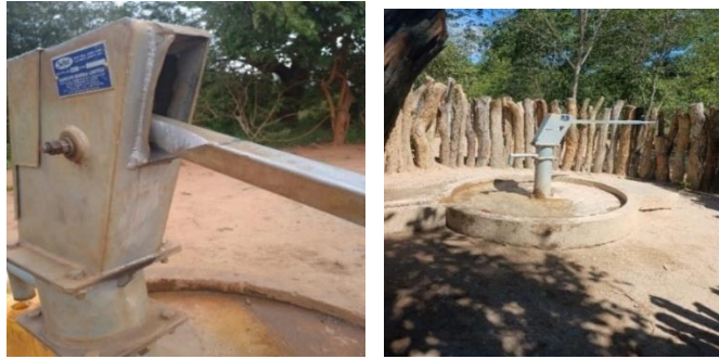
Pump handle eroding at Nemfwe Pump at Sikubomba
