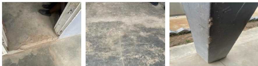
Floor cracks and poorly plastered pillar
