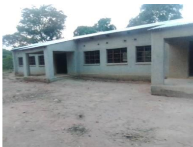
Incomplete classroom block
