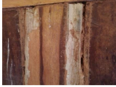
Door Exposed to Termites
