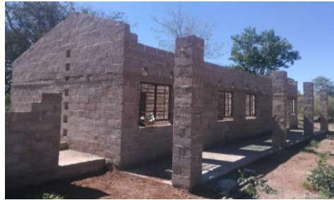
Delayed completion – Lunungu Maternity Annex
