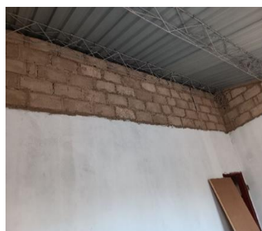
Incomplete plastering works
