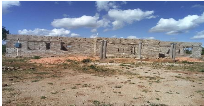
Incomplete Police Post at Kagoro
