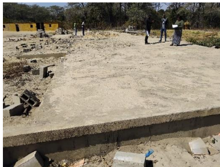
An abandoned slab eroding at the centre
