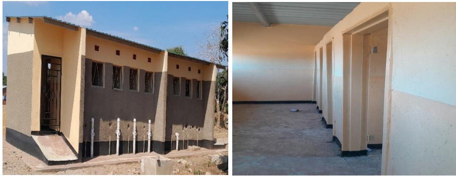
Incomplete ablution block
