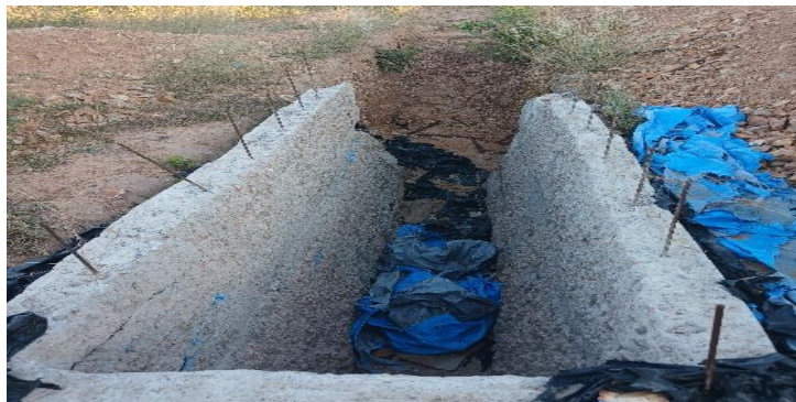
Incomplete Dip Tank in Siatambo
