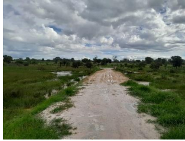
Incomplete works at Moboshi bridge
