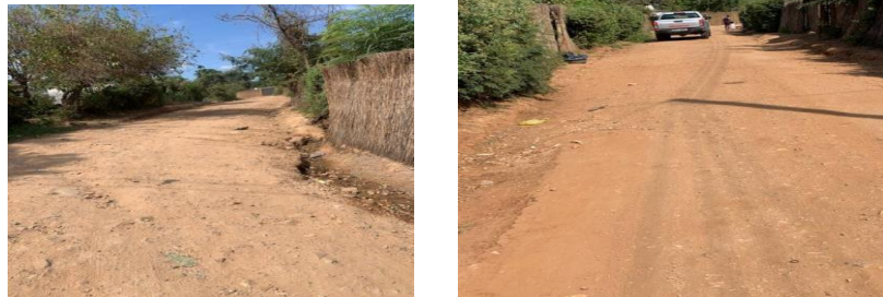
Washed way side drains and spot gravel
