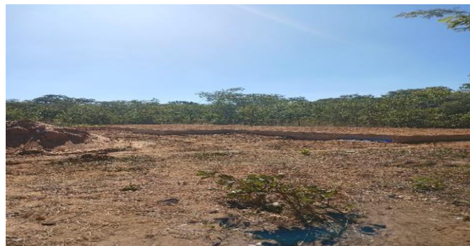
Incomplete 1x3 CRB at Sichikwekwe Community School
