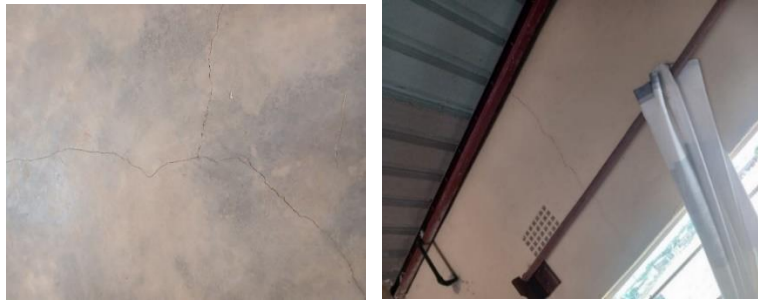
Cracks on the Wall and Floor
