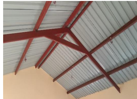
Electrical installations not installed
