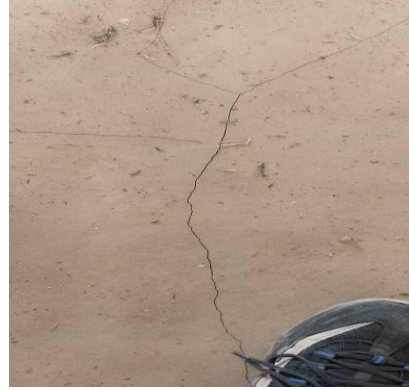
Cracked Floor in the Classroom
