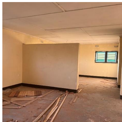
Installation of Bunker Beds not done
