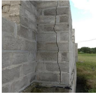
Cracked wall 1x3 CRB
