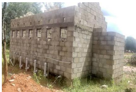
Incomplete water borne toilets
