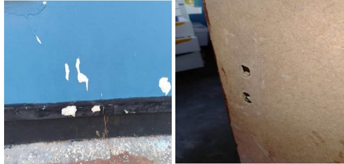
Paint Peeling off
