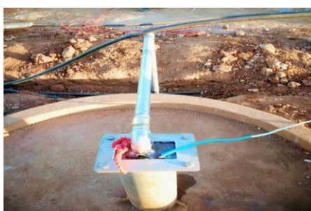
Incomplete water system at Simbulo Primary School
