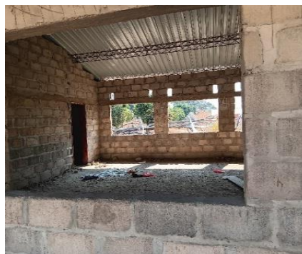
Windows and air vent not fitted
