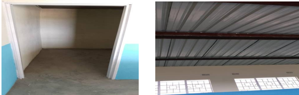
Strong Room Door and Ceiling Board not Fitted
