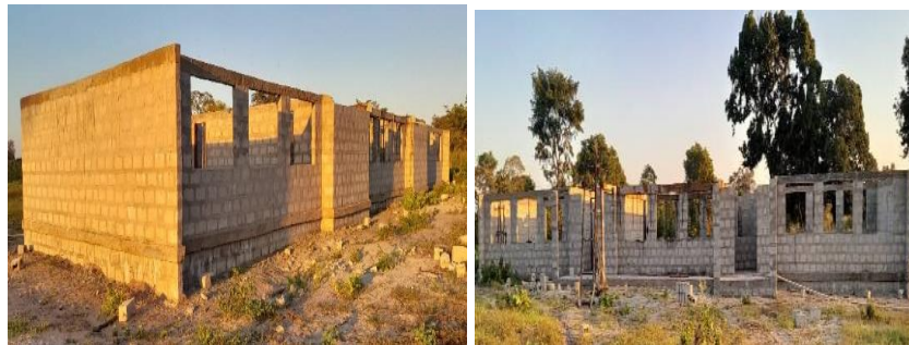
Incomplete and stalled works
