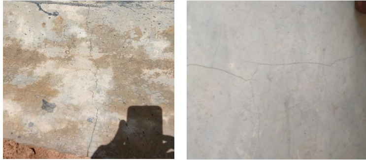
Cracks on the Spoon Drain and Floor
