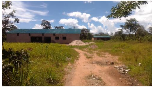
Incomplete health post and staff house
