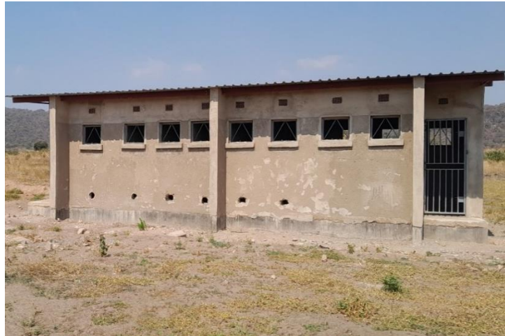
Incomplete Ablution Block
