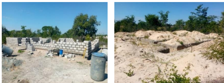
House No. 01 at window level House No. 02 only foundation trenches had been done
