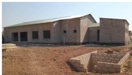
Incomplete Chalokwa Rural Health Post
