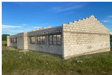
Uncompleted 1x2 CRB at Chilombo School
