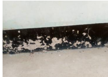
Paint peeling off
