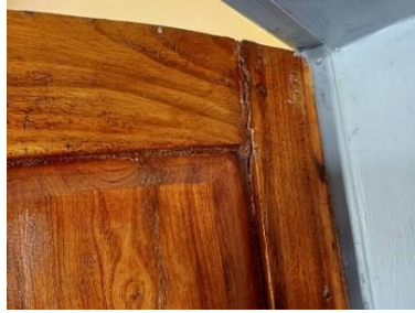
Hard wood door with cracks
