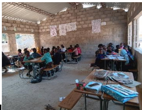
Learners in an Incomplete Classroom
