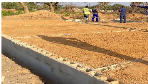
Incomplete Chishikishi Rural Health Centre
