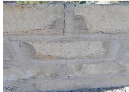
Cracked wall of 1x3 CRB
