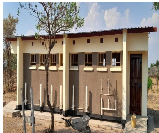
windowpanes not fitted
