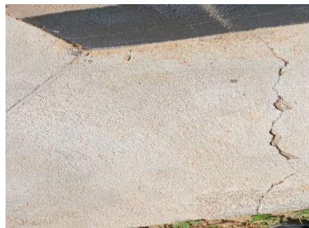
Cracks on the Apron
