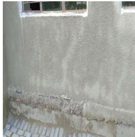
Peeling off plaster
